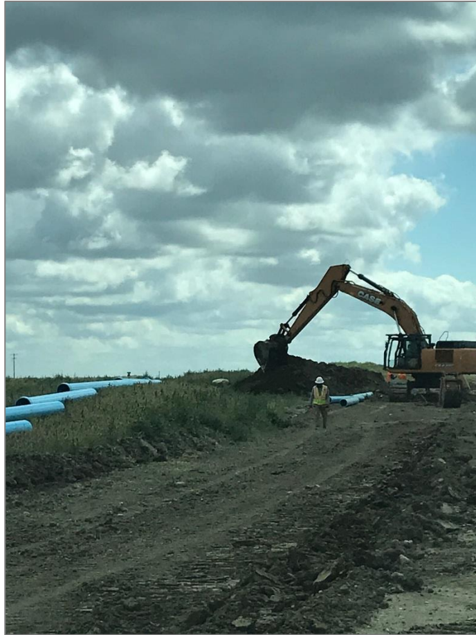
XWA On Site Water Distribution
