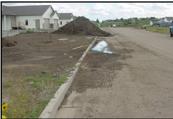
Stockpiles cannot be placed in streets or ditches
